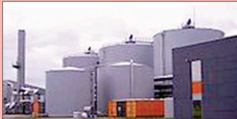
Fig: Anaerobic digestion in a treatment plant of Germany.
